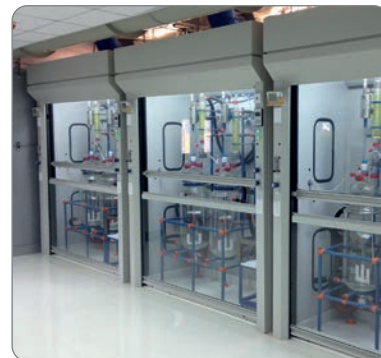
An installation of six 30 litre jacketed reaction systems in Shanghai, China
